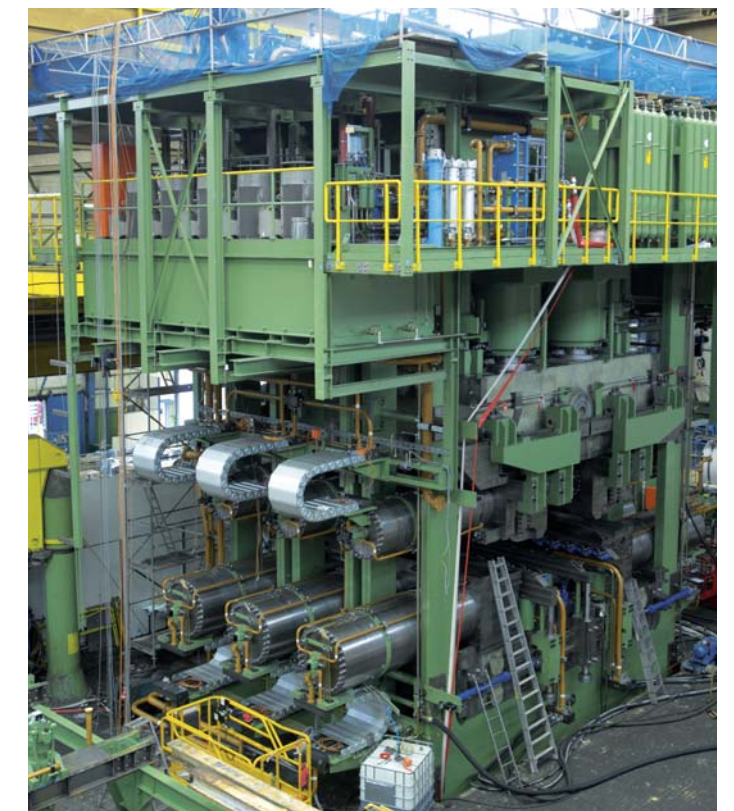
Ready for commissioning
